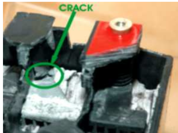
Fig. 4. View of damaged battery without lid [9]
